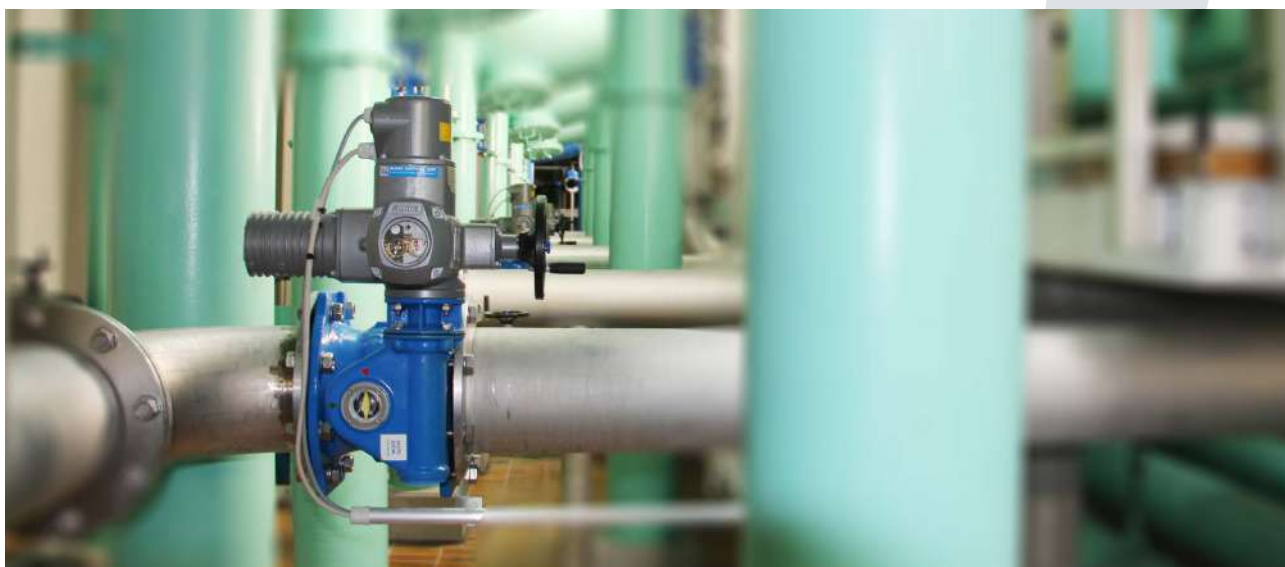
Installation at the drinking water treatment plant in Sindelfingen, Germany
